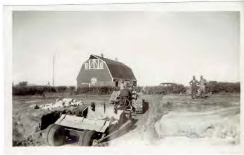
ph698(1) Florence Boyne Fraser 15-16eca. "This is the government outfit taking the dirt out of the basement June 1946"
