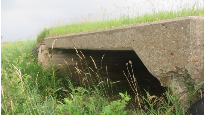
Additional Structure #17 – Perth Line 86 BCI – 26 (Poor)
